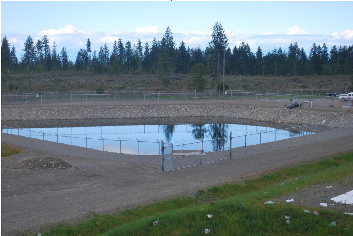
Leachate Equalization Pond
